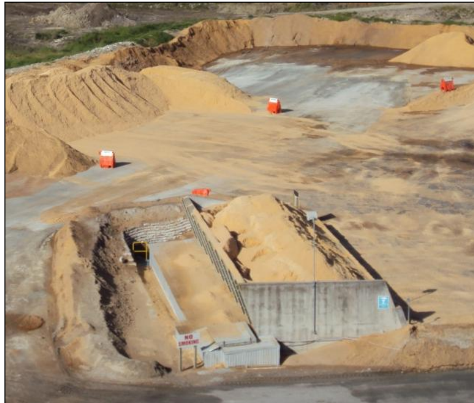
Wood waste loaded into the hopper from the storage pad, ready to be conveyed to the calciner, and then fed into the kiln.
