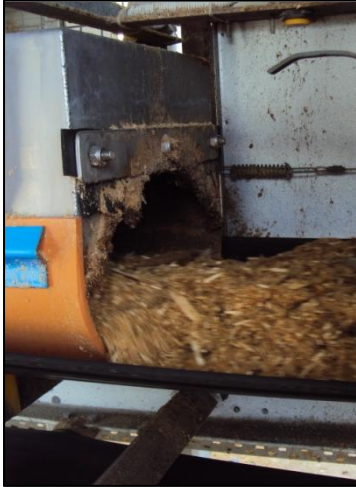
Wood waste feed system.
