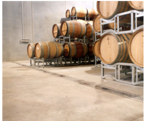
Figure 3. Wine is mildly aggressive to concrete. Extended service life and improved hygiene can be achieved with the use of Microsilica 600.
